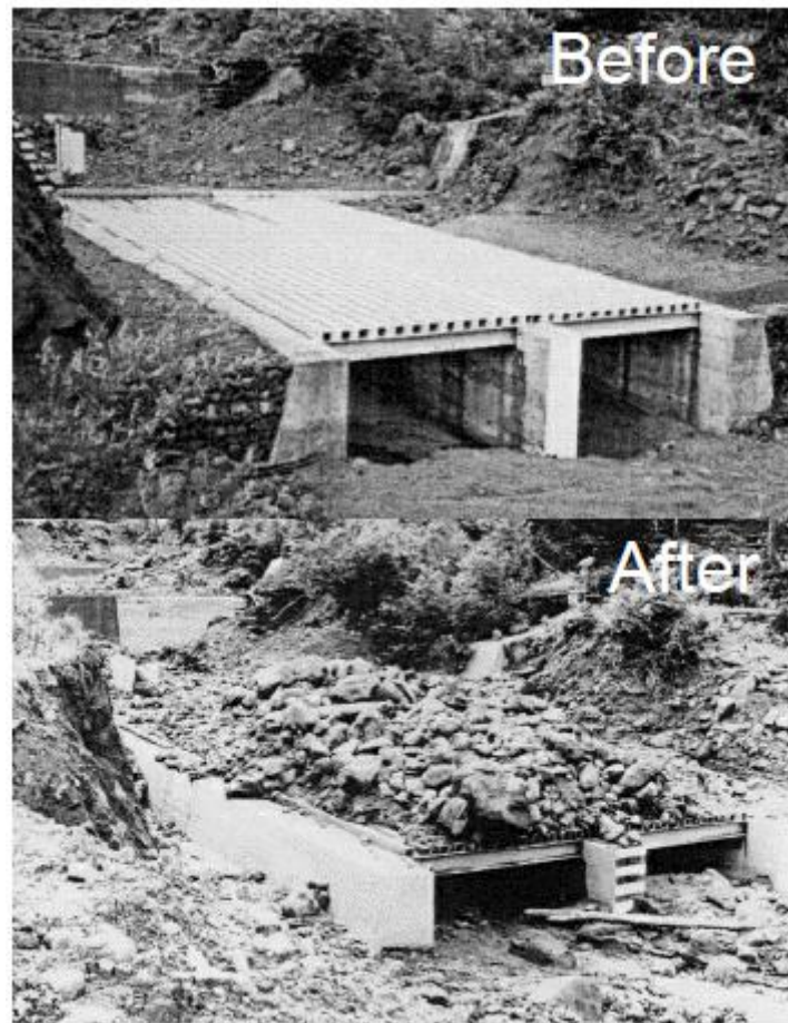
Figure 3.7 Pictures of a permeable rack, before and after the occurrence of a debris flow in the Kamikamihori Valley, Mt. Yakedake, Nagano Prefecture, Japan (Cascini et al., 2016).
