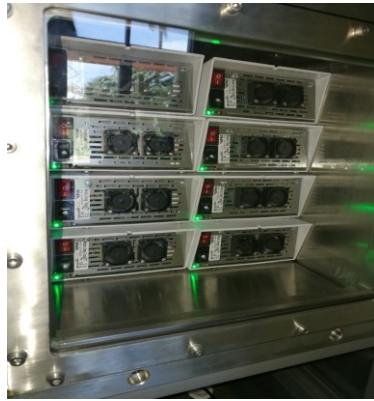
Figure 1. 9 LVTC with eight MONICA node under laboratory calibration procedure.
